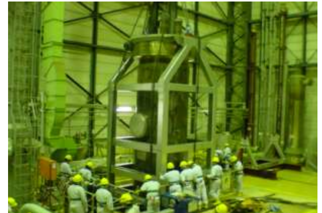
Lift-down inside Pit of Maintenance Building
